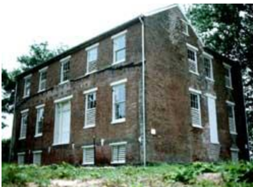
This building has been successfully mothballed for 10 years because the roof and walls were repaired and structurally stabilized, ventilation louvers added, and the property maintained. Photo: NPS files.
