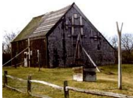
Buildings seriously damaged by storms or deterioration may need to be braced before architectural evaluations can be made. Photo: John Milner Architects. Photo: NPS files
