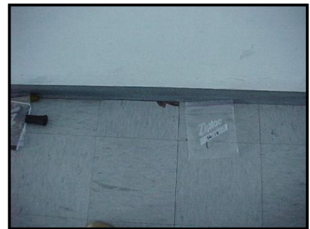
Figure 25: Vinyl Floor Tiles
