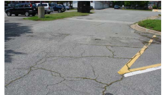
Figure 7B-2: Cracked pavement requiring repair
